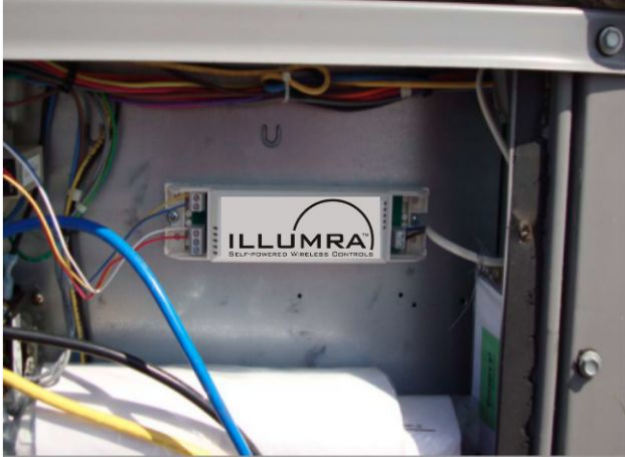
Figure 1- ACSVR installed inside control panel of RTU.
