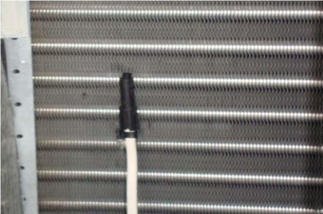
Figure 3- Sensor attached to supply side of evaporator.
