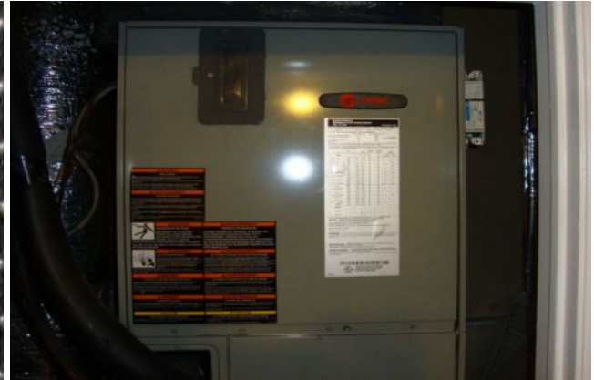
Figure 4- ACSVR attached to exterior wall of air handler.
